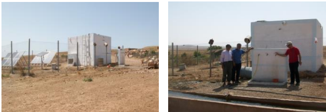
Photo 2: Pumping PV installation (2 kW), in the framework of UNDP and BTC projects in Douar Zragta of the Issly rural commune of Oujda Morocco
