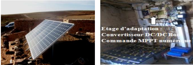
Photo 1: lighting PV Installation (2 kW), in the framework of PNUD and BTC projects in Douar Zragta of the Issly rural commune of Oujda Morocco
