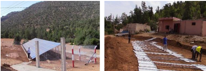
Photo 3: Water pumping plant (15 kW) in the framework of the NIHD, for domestic use (20 homes) and irrigation of 100 hectares in the rural commune of Tafoghalt. (Berkane).
